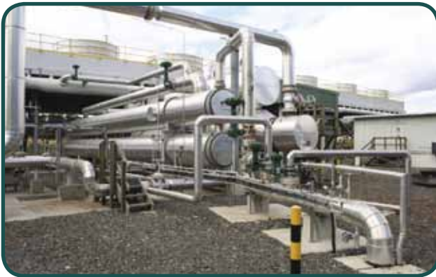
The GDL plant at Kawerau.
