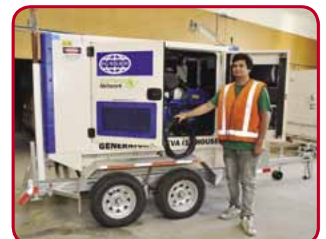
Eastland Network engineer Mikaere Ngarimu with the new mobile generator.
