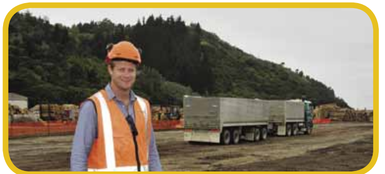
Where it all starts....project development manager Marty Bayley stands near Eastland Port's biggest ever capital investment project - a $15 million asphaltting of the main log yard area.
