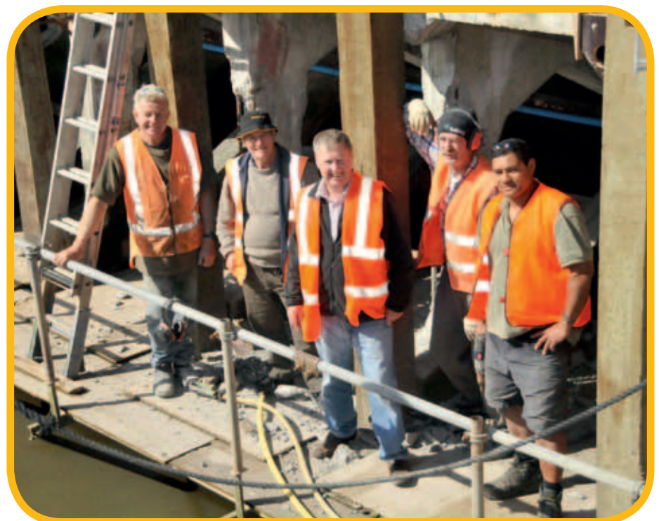
Fine work calls for team work.... (from left) safety supervisor Chris Olsen, Eastland Port Neil Burgess, Graeme Ritchie, Len Rickett and Lindsay Pihema at work on the million dollar refurbishment of the wharves.
